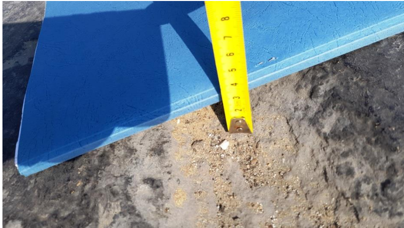
Figure 3. The depth of maximal pavement's damage after steel scrubs handling
