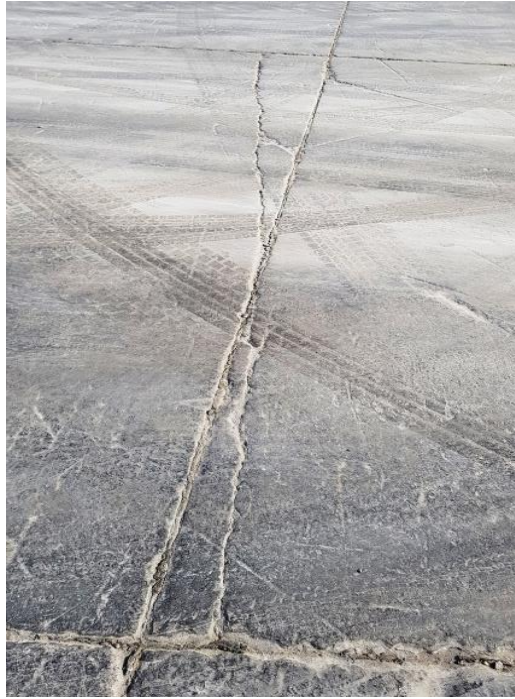
Figure 6. Cracks next to the saw cut joint
