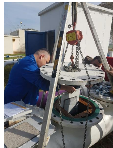
Figure 4. In-situ exposure of the cement based lining conditions inside the functioning water-supplying
